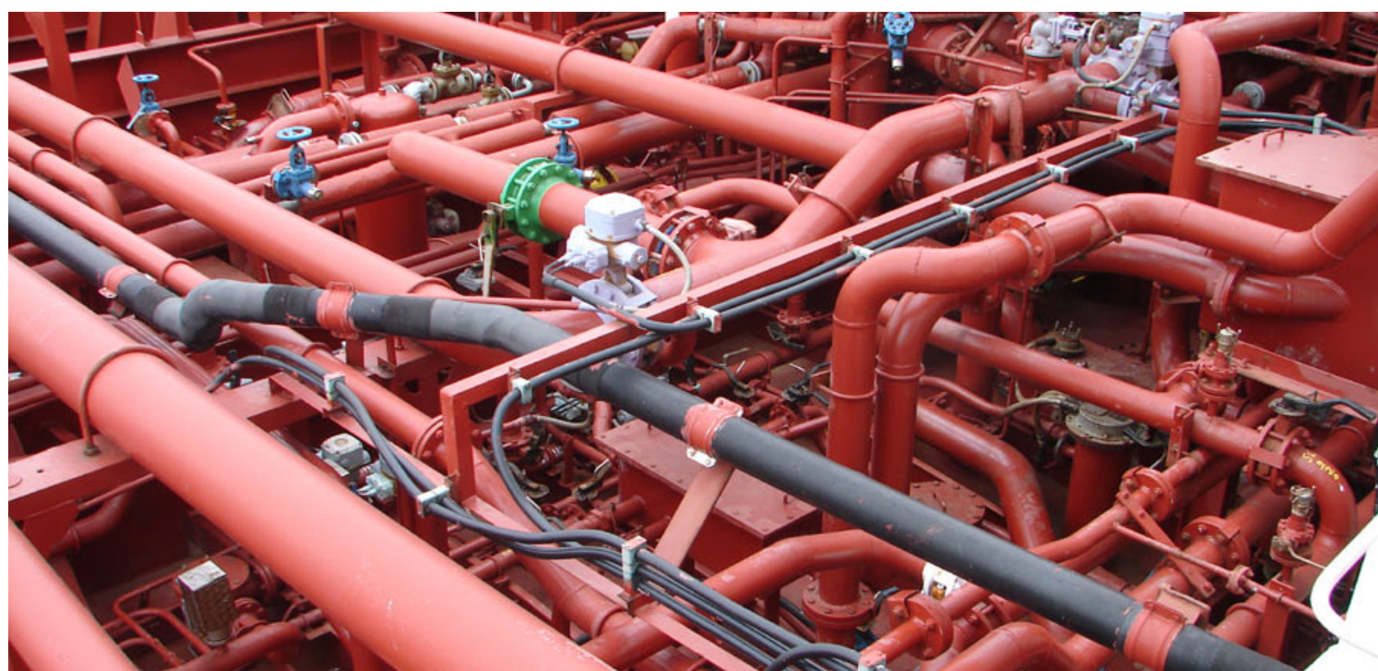
FIGURE 1. Piping systems on an oil/chemical tanker. Image licensed under CC BY-SA 3.0 via Wikimedia Commons.
