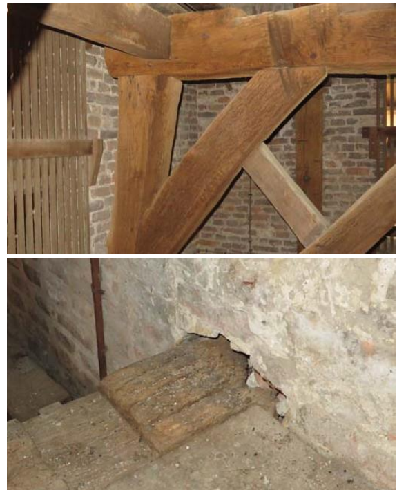
Figure 1. Wooden beam end (bottom) as part of the internal construction (top) of a church in Beusichem. The end disintegrated and is not connected to the wall anymore
