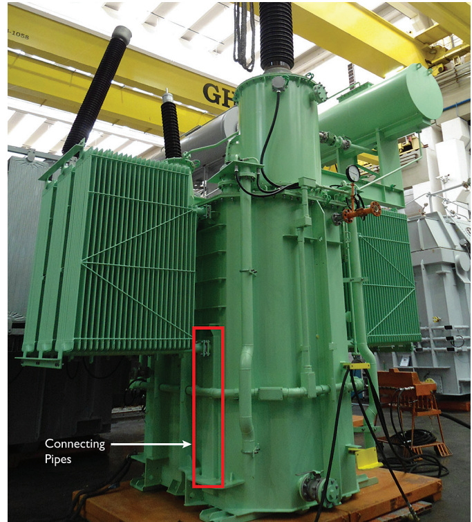
FIGURE 1: Shunt reactor. In the original design of the oil circuit the radiator is connected to the tank by pipes enclosed in rectangular boxes welded to the exterior of the reactor.
